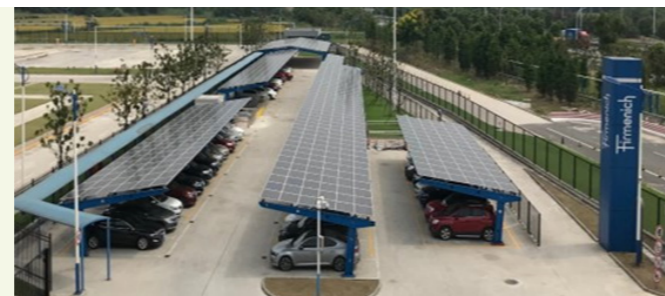
Solar photovoltaic panels
